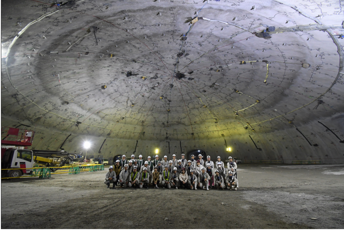
Figure 6: Excavation of the dome section of the cavern that will house the Hyper-K detector, completed on 3rd Oct. 2023. The dome is 69 m in diameter and 21 m in height.
