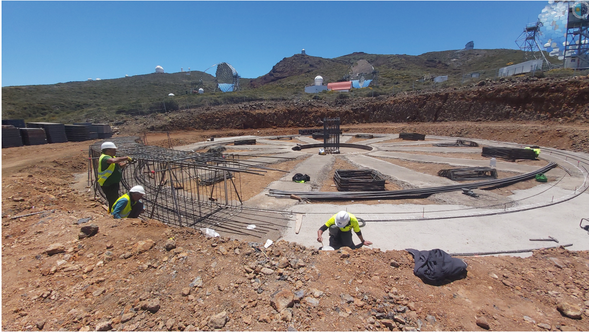
Figure 5: Status of the civil works at the LST-4 site, as of June 2023. Courtesy by Javier Herrera (IAC).
