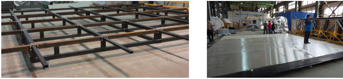
Figure 3: Left: the TT wall supporting structure. Right: a TT wall is mounted on the structure.
