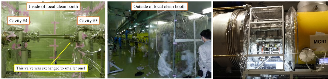
Figure 3: Local clean booth used for beampipe connection in STF tunnel (left and center), and high-quality local clean booth and particle counter used in E-XFEL at DESY (right).
