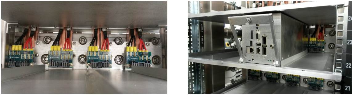
Figure 6: Left: Power bars with power backplanes attached via cables. Also visible are the quick-disconnect couplings (female parts) for in- and outlet. Right: A brick (of height 3U) is being inserted into its slot.
