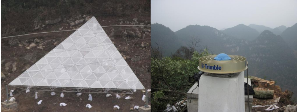
Fig. 8 At the FAST site, a full-scale reflector element was set up (left panel); the basic control network for the measurement system established for use (right panel).
