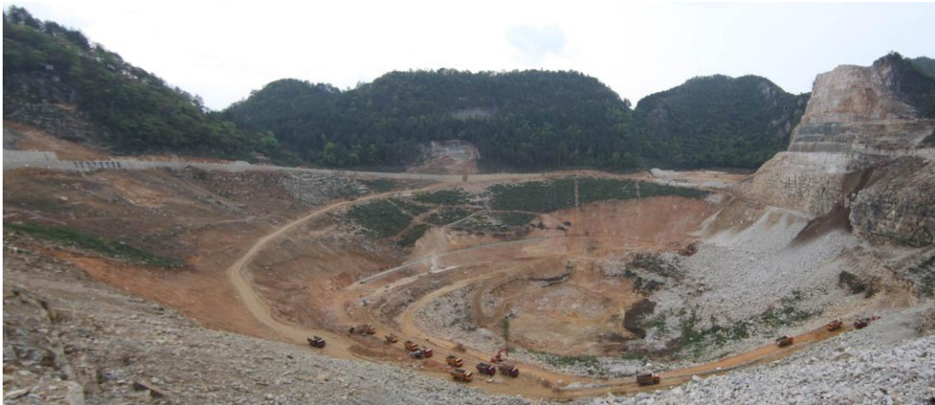
Fig. 7 A snap shot of the Dawodang depression in April 2012: all the earthworks have nearly been done at the FAST site.
