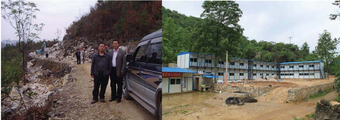
Fig.3 A path connecting the county road and Dawodang depression under construction (left panel), and site accommodation for temporal use built up (right panel).
